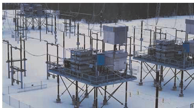
Fig. 4 One segment of a 301 Mvar 400kV - 50 Hz series capacitor bank at Keminmaa substation in Finland.
