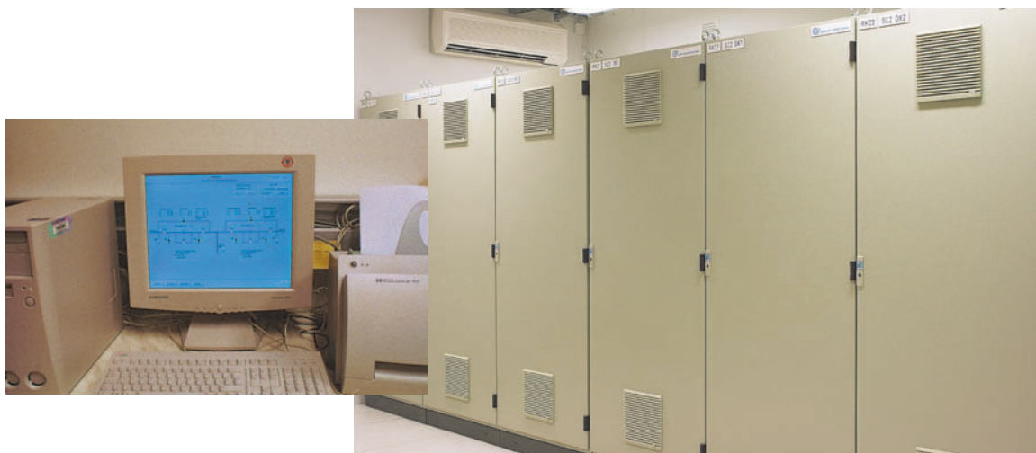
Fig. 6 Typical arrangement of the control cubicles and MMI in the control building.
