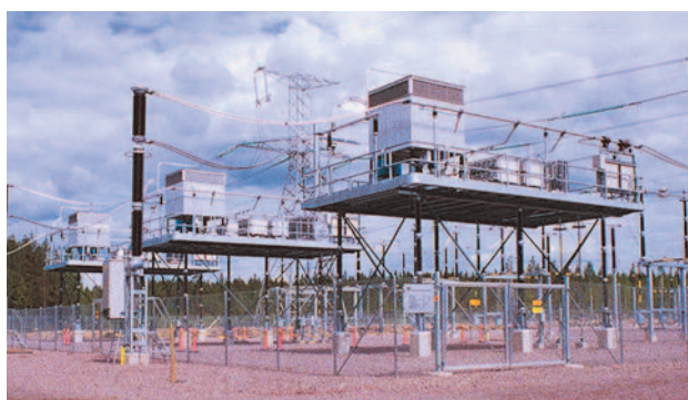
Fig. 5 Series capacitor bank, 105.9 Mvar 400 kV - 50 Hz, at Uusnivala substation in Finland.
